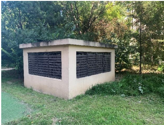
155 地块排风竖井 (3)
